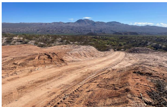
SunZia right of way preparation in New Mexico – 3CE didn’t tell the Operations Board about the Tribal opposition.
